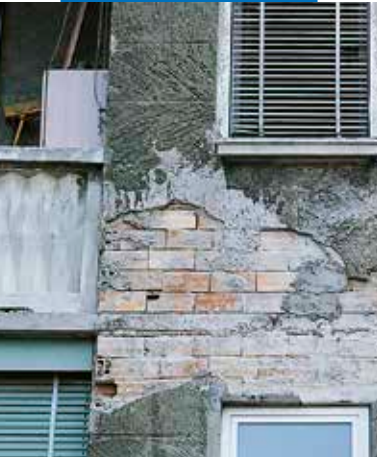
Degraded building façade in need of repair
